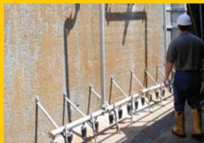
The assemblies can be lifted out, inspected and replaced without having to dewater the channel. The cradle brackets provide a guide when reconnecting the assembly.
