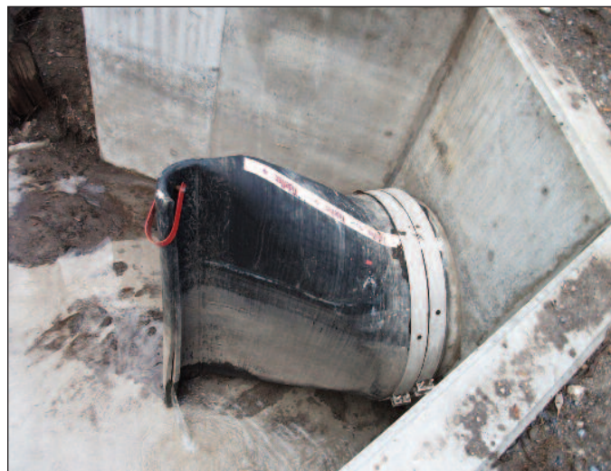
A Tideflex® TF-1 Check Valve installed on the River Barrow to protect Carlow from flooding.
